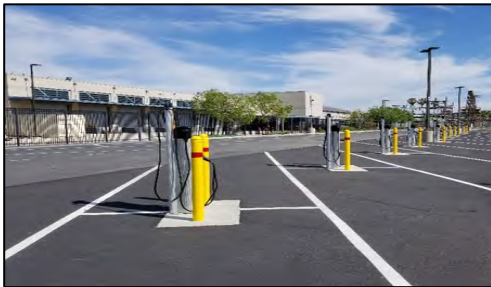
EV Charging Stations, PCC - Lot 10
