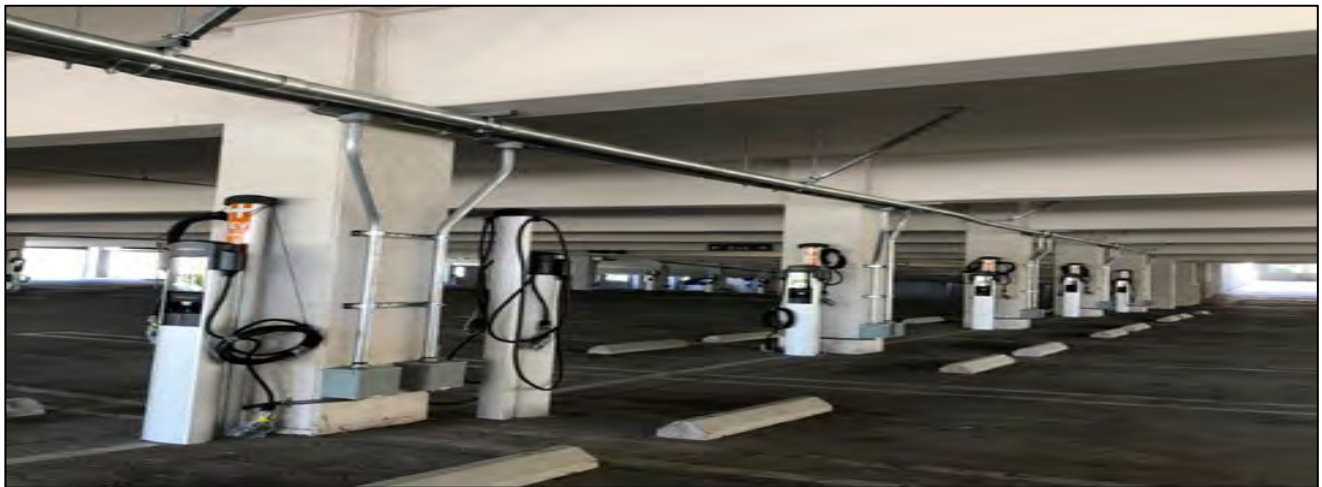
EV Charging Stations
