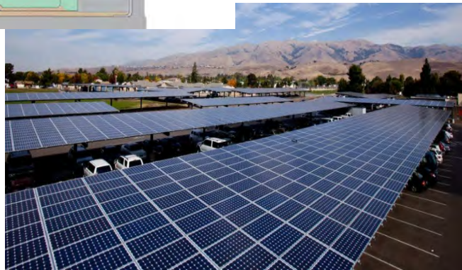
Solar Panel Canopies - PCC
