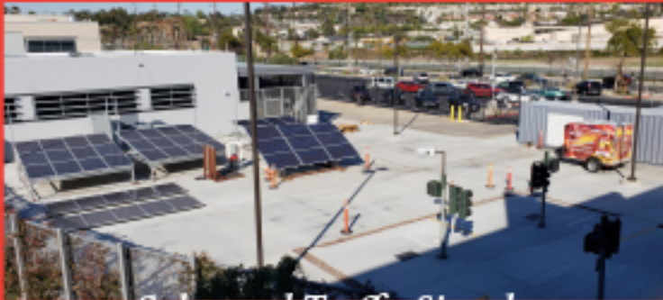
Solar and Traffic Signals
