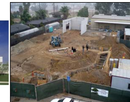
Central Plant – PCC
